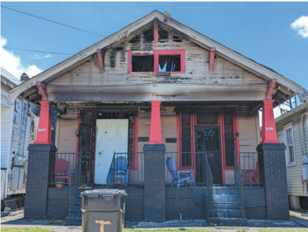
Exterior photos showing the charred remains of Winchester's former New Orleans home after the June 5 fire.
