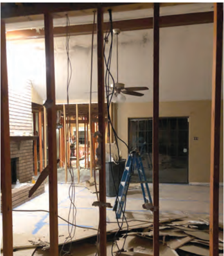
Home damaged following Hurricane Ida.
