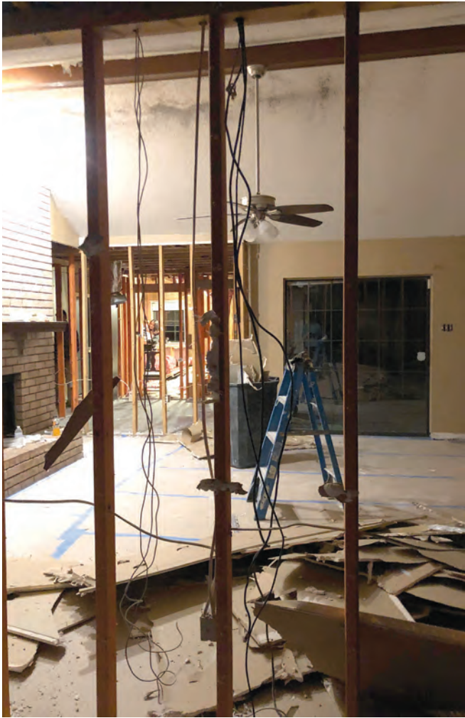
Many St. Charles Parish homes are still gutted following Hurricane Ida.
