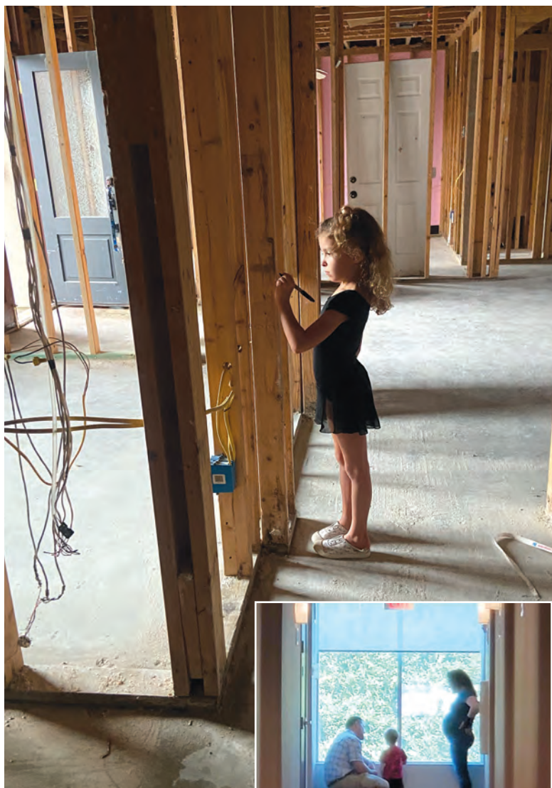
Still rebuilding nearly a year after Hurricane Ida – as well as being pregnant and evacuating during the storm – are all too common stories for many St. Charles Parish residents.
