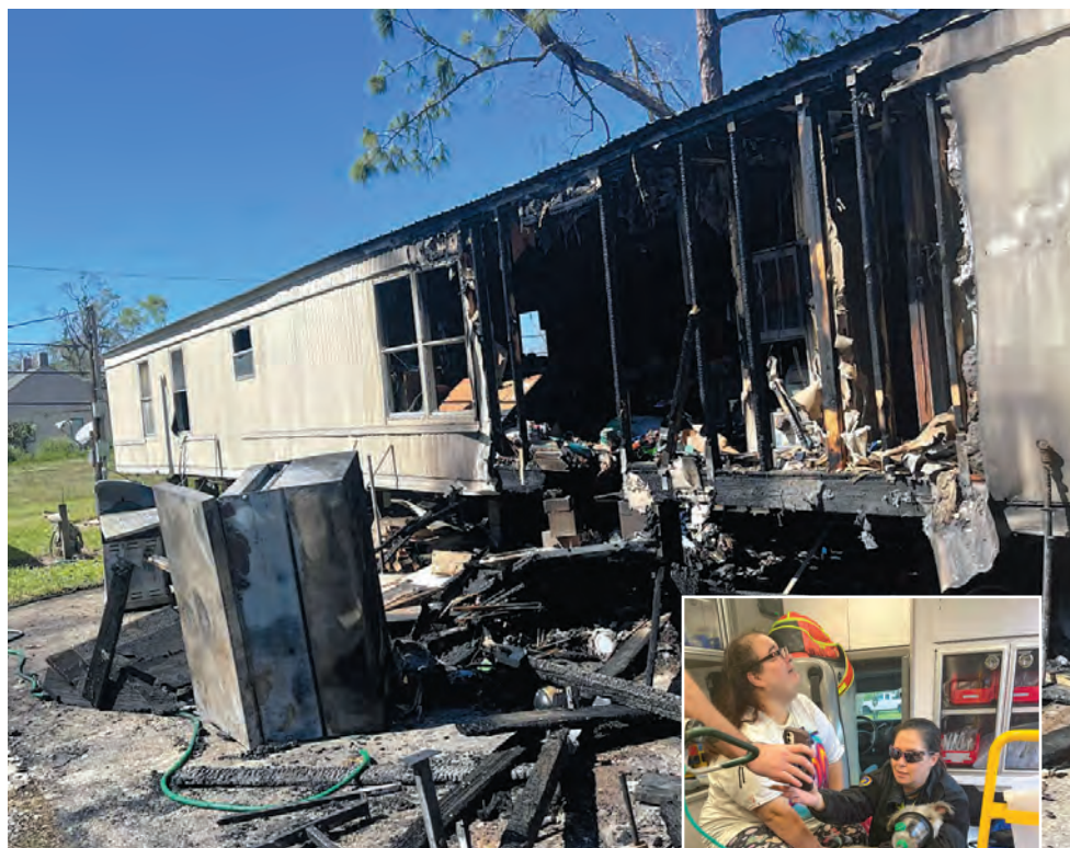
The home of Cory and Stacey Trosclair following a March 30 fire. The couple and their roommate were forced to find an escape and received medical treatment.
