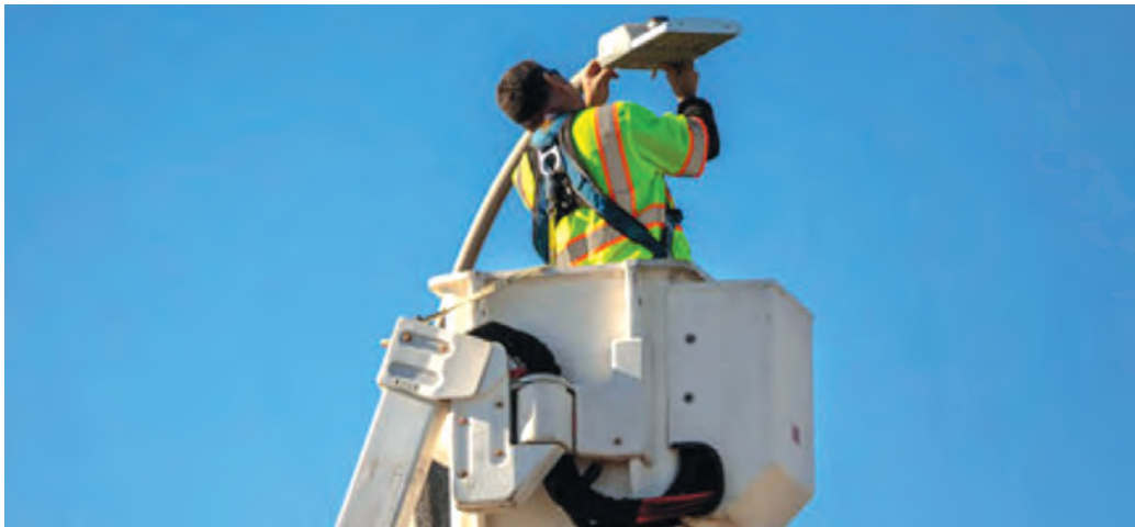
Thousands of parish street lights were damaged during Hurricane Ida.
