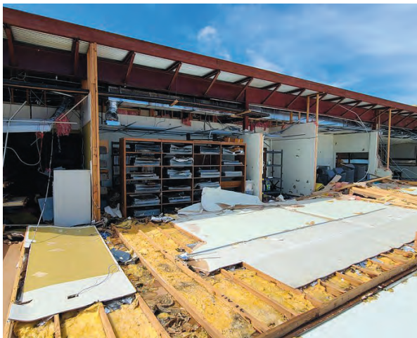
West Regional Library following Hurricane Ida.
