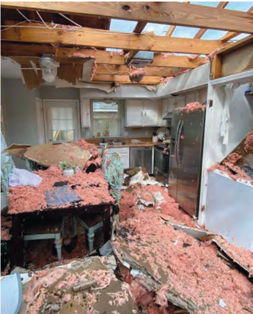
(Top) The Wards embrace under their new roof. (Above) The storm took the roof completely off the house and the insulation and ceiling caved in.
