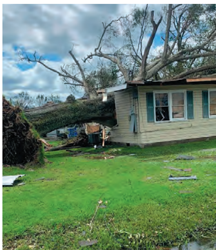
The Nichols' home after Hurricane Ida caused extensive damage.
