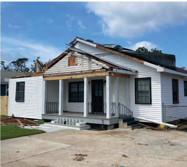
Damage to New Sarpy home caused by the winds of Hurricane Ida.
