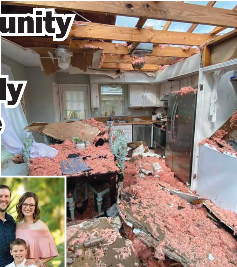
Home of Josh and Kati Ward following destruction caused by Hurricane Ida.
