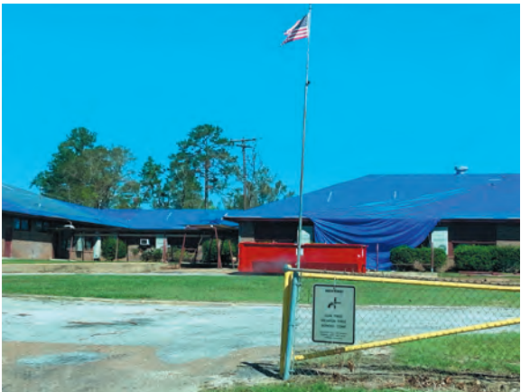
A school in Allen Parish damaged by Hurricane Laura.
