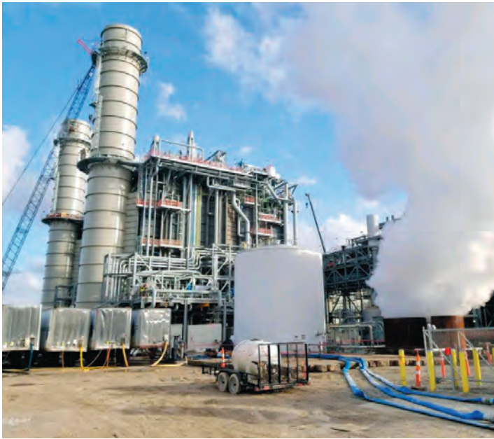
Entergy’s St. Charles Power Station conducting a “steam blow” test.
