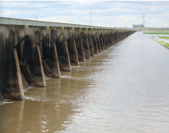
The Bonnet Carre Spillway flooding from high waters in Norco.
