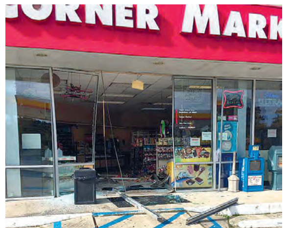
Corner Market in Destrehan after a car drove through the front of the building.
